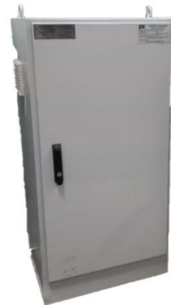
FRTU PANEL ENCLOSURE
