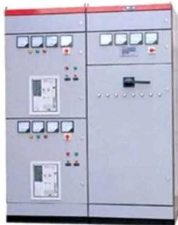
ELECTRICAL & INSTRUMENTATION PANEL
